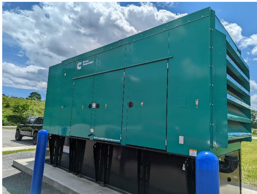
Figure 12 Existing Diesel Generator Providing Power to the Depot During Outages
